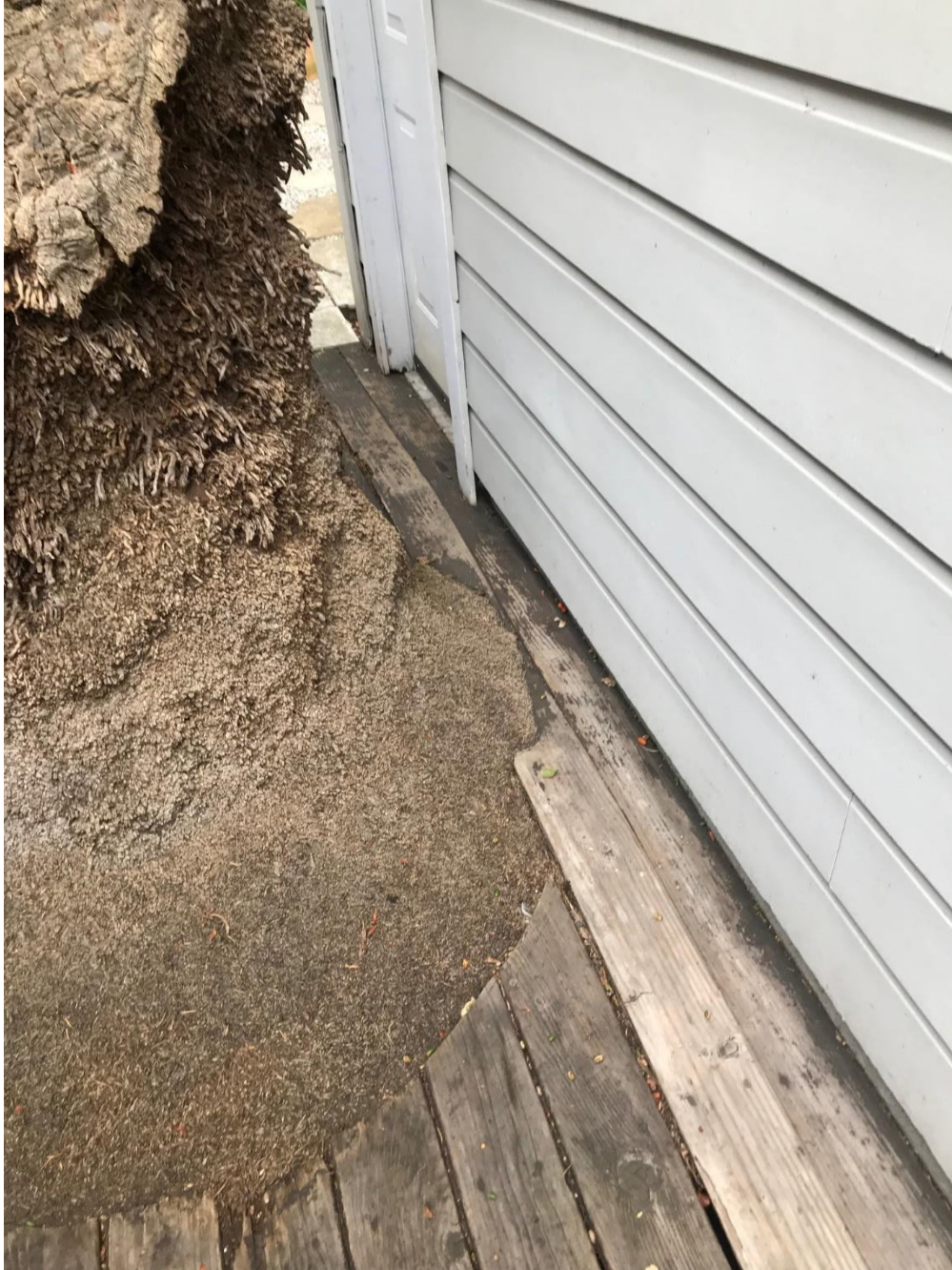
PHOTOGRAPH 3 - Subject tree showing its trunk location in direct proximity to garage foundation.
